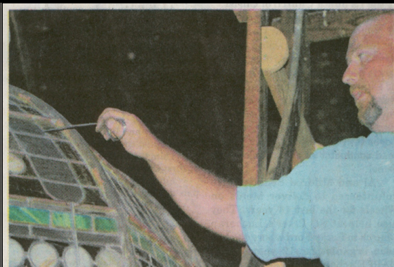
Robert Bohannon, foreman with an Associated Crafts crew, points to a portion of repairs he and his crew have completed on the stained glass dome at the CommUnity Presbyterian Church in Rocky Ford. (Photo By Susan Pieper)
